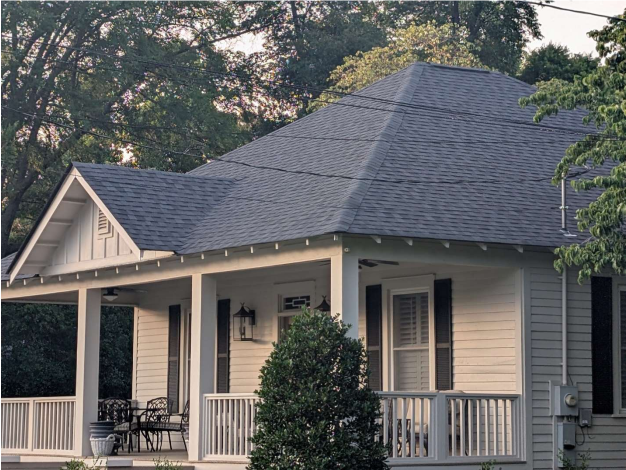
Roof of 906 Washington Street with ridge vent (This roof was replaced in the past year)
